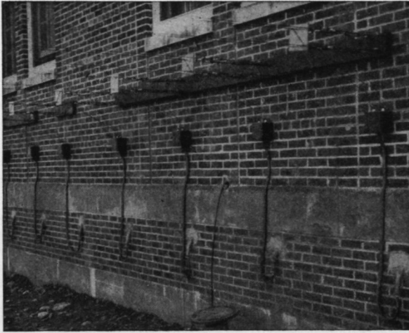
FIG. 4.106. Detail showing the feeders for a receiving installation using four-wire cross-connected open-wire feeders terminating at a building and entering through coaxial feeders. The wide-band high-frequency balance to unbalance transformers are in the weatherproof black boxes on the building. (Photograph courtesy of Royal Canadian Navy.)
