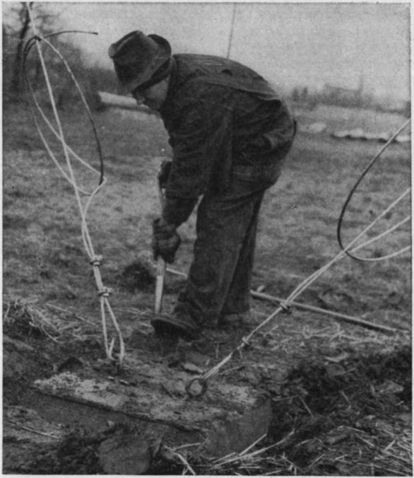
FIG. 3.108. Detail of guy anchor for the pole supports of a high-frequency antenna system.
